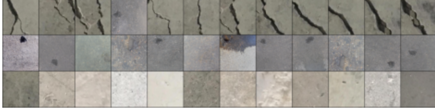
Fig. 6. The visualization of the Road Surface dataset, which contains cracks (the first row), potholes (the second row), and normals (the third row). As we can see, each class contains several confusing samples, e.g, the fourth one, the third one, and the second one for each class, respectively. The PCMO method aims to detect confusing samples, reducing the classification risk.
